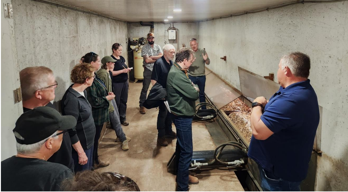
Prince County Hospital woodchip heating system with owner Dick Arsenault of Atlantic Bioheat Inc. – May 12, 2023
