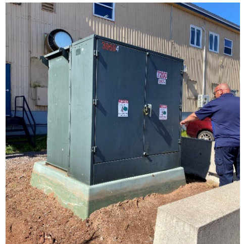
Figure 3. Newly elevated electrical box following Post-Tropical Storm Fiona. Image from ICF.
