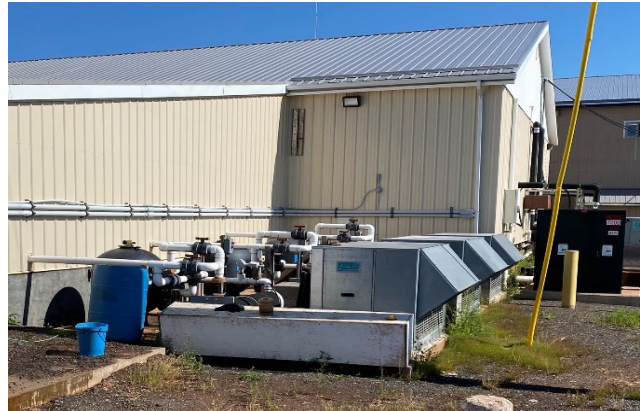
Figure 2. Critical electrical equipment at Acadian Supreme. Image from ICF.
